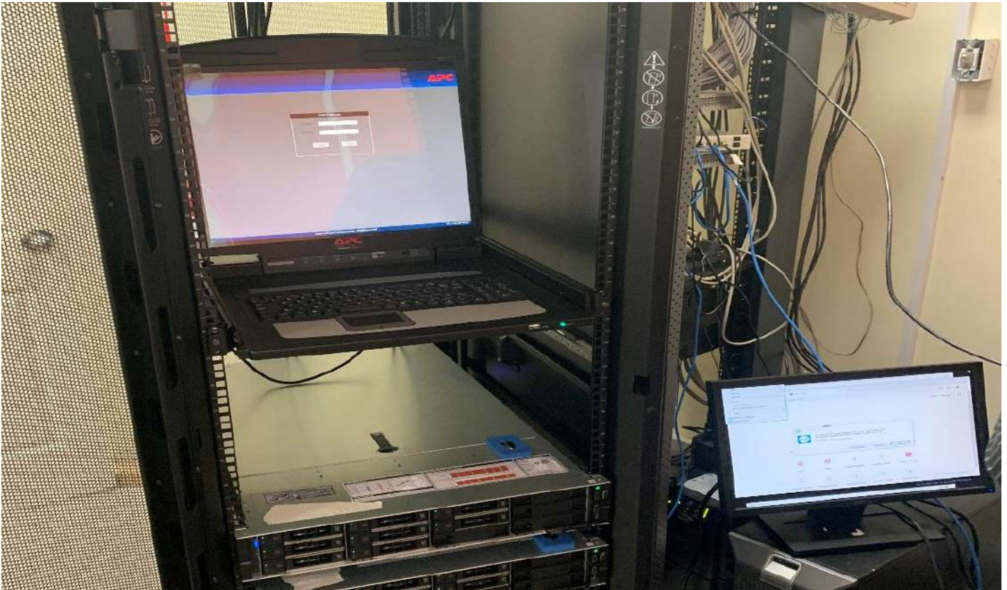
Console and associated components
