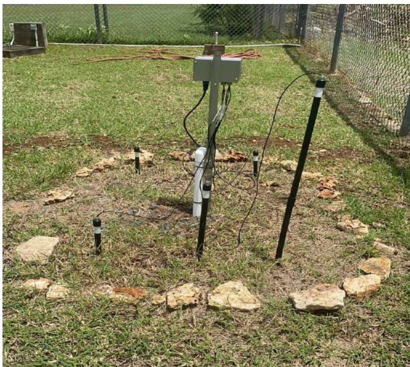
Application on a cellphone IntelliSense System at MET Services Tobago
