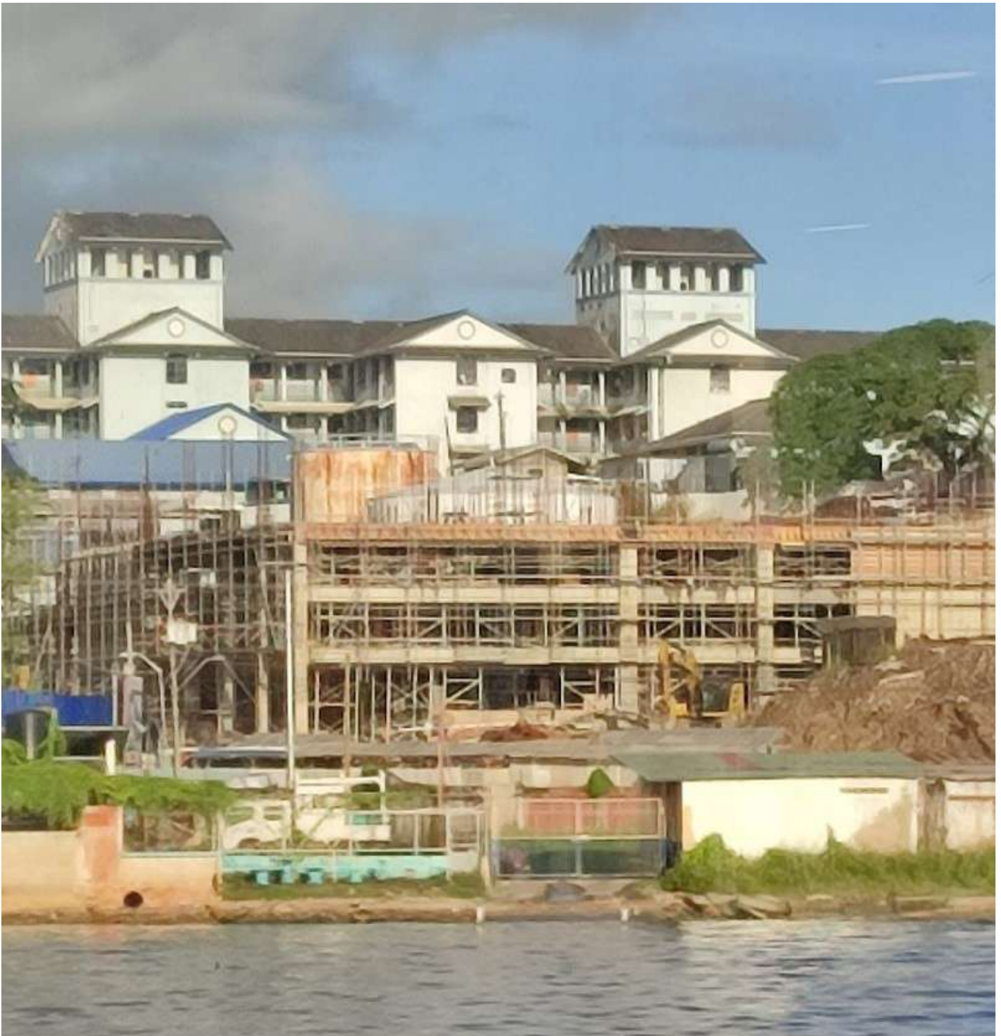
Construction of Multi-Storey Carpark at the San Fernando General Hospital View from the Gulf of Paria of the construction of the San Fernando General Hospital's Car Park
