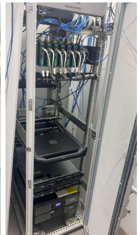
(G.O.E.S) Ground Station Satellite Monitoring Station 2
